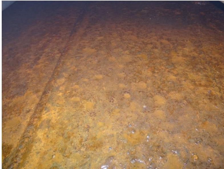
Figure 4.1.2.5(6)①b Typical pitting corrosion of inner bottom plating in cargo oil tank
