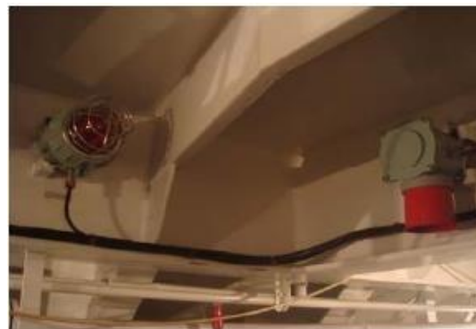
Figure 5.5.3.1(1)(4) Explosionproof lamp and explosionproof motor
